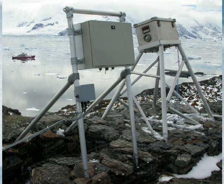
New camera (nearest) alongside old at Signy. Rock filled gabions provide anchorage for the structures.
